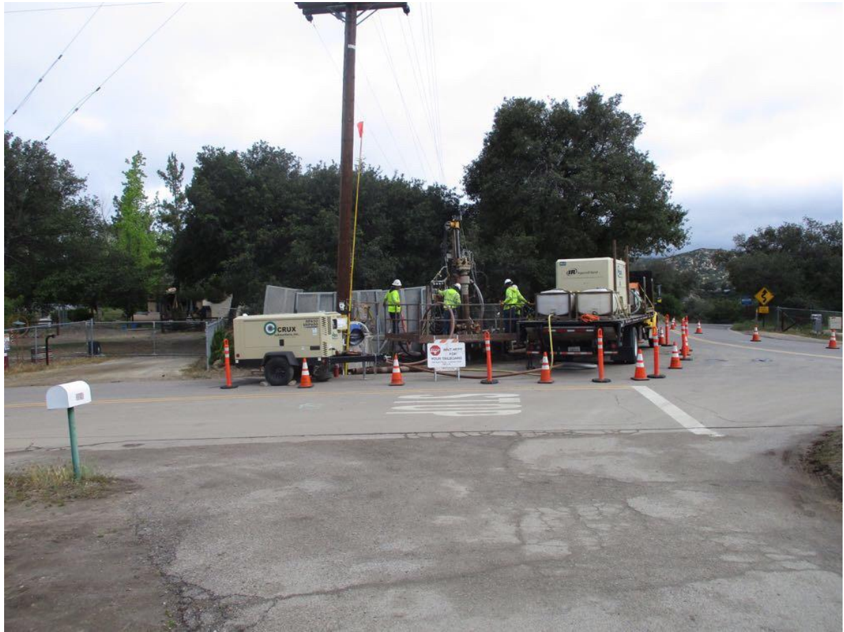
Photo 2: During micropile drilling at Pole Z273069 (TL 629A), a noise barrier was erected to minimize disturbance to adjacent residents in accordance with MM NOI-1.
