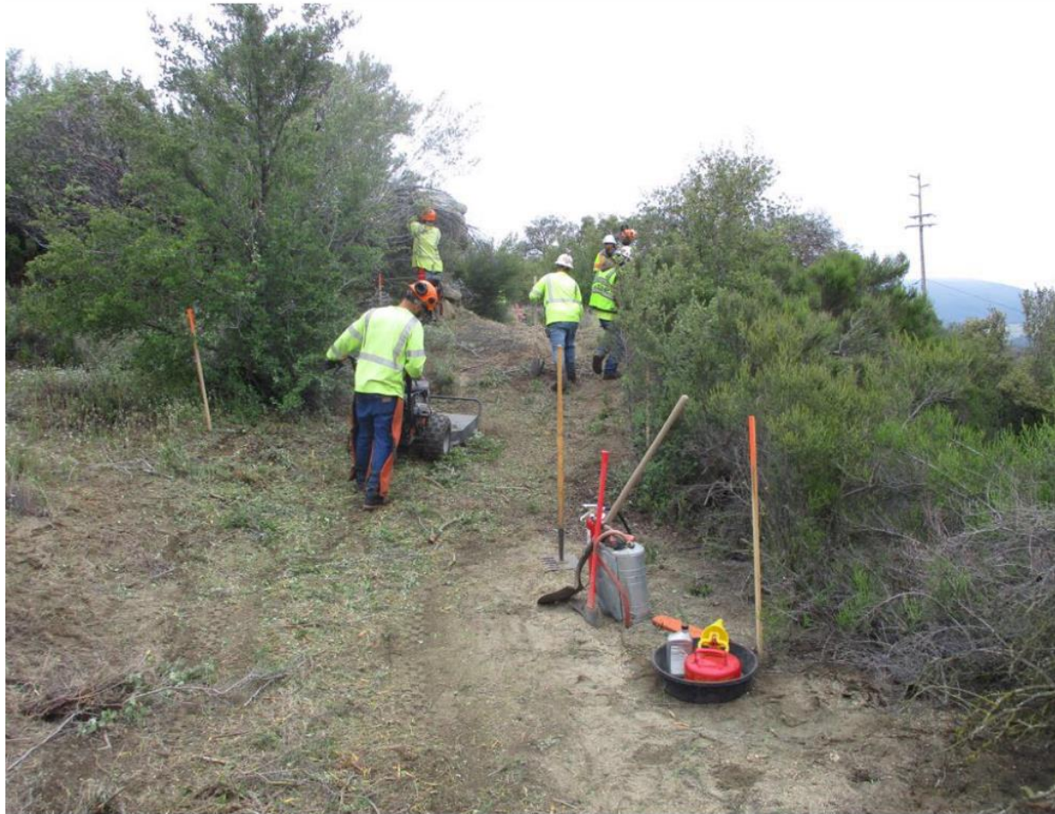
Photo 3: A crew was observed clearing vegetation along access to P258376 (TL 629A). A set of fire tools was staged within 50 feet of clearing work in accordance with the CFPPP, and fuel was staged in a drip pan in accordance with the SRNP.
