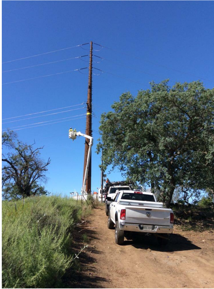
Photo 5: A construction crew was observed conducting dead-end activities (overhead work) on a line at Pole Z118027 (TL 682). The crew was observed performing work within the access road and only in approved work limits in accordance with MM BIO-1.
