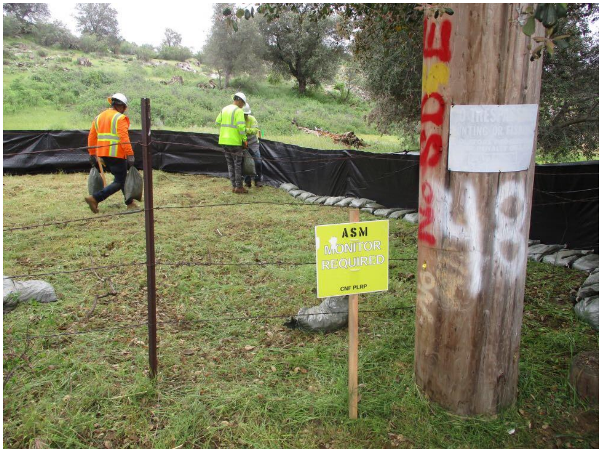
Photo 1: A construction crew observed installing a silt fence at a pole site at TL 629A in accordance with the Erosion Control Plan and SWPPP. Securing the silt fence was performed by placing gravel bags on the ground flap to avoid ground disturbance at the site. Archeological and Native American monitors were present on site during the work, and ESA signage was present in accordance with Attachment A of the HPMP.
